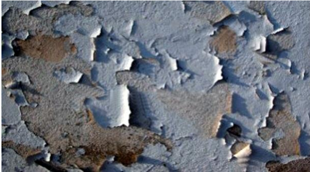
Paint peel off
